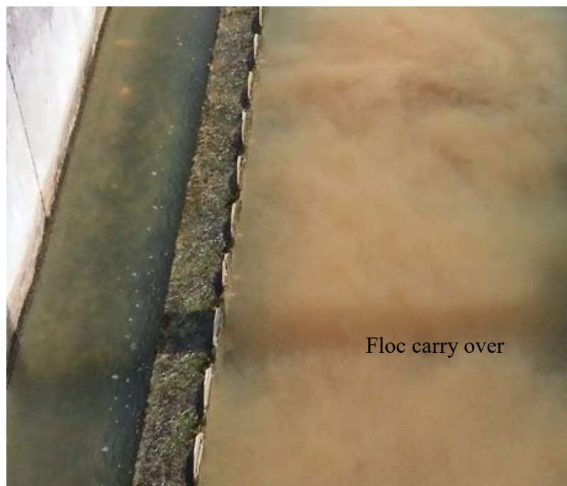
Figure 1.7 Floc carry over during the water treatment process at a sedimentation tank (brownish colour) – the main cause for clogged filter. The production output will decrease, and the in-plant losses will increase.
