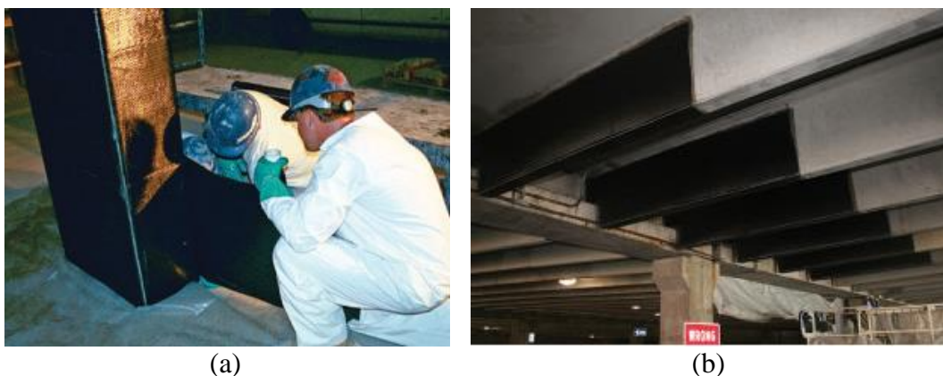
Figure 1.2 FRP sheets wrapped around RC parts to enhance shear and flexure strength; (a) columns and (b) garage beams (Alkhrdaji, 2015)
