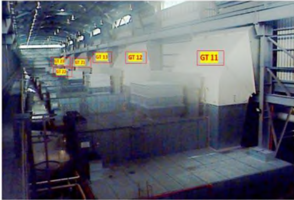
Figure 1.2 GT11 at GT Hall
