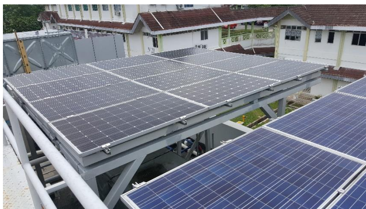
Figure 1.3 Solar panels at School of Chemical & Energy Engineering, N01a, University Technology Malaysia, Johor Bahru (2018)
