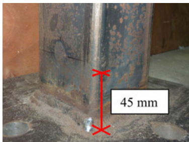
(c) Deformation of SHS-20 (left face)
