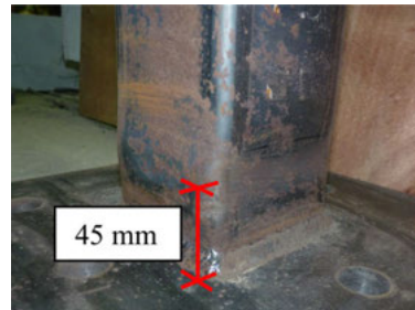
(b) Deformation of SHS-0 (right face)
