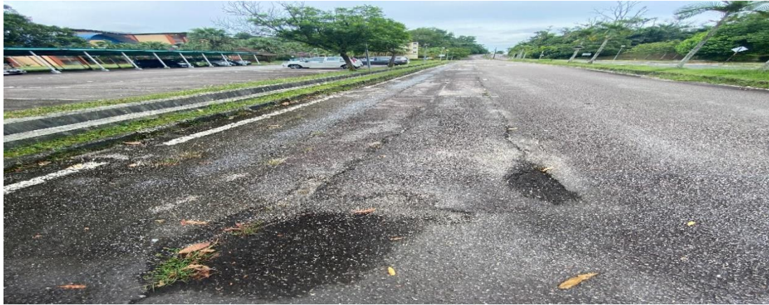
Figure 4 Poor condition of road at UTM Technovation Park
